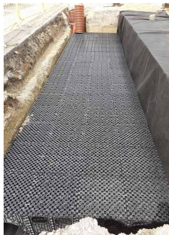
Faskiner under regnbæd
